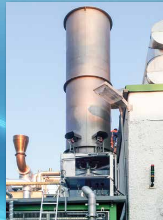
↑ Wood gas flare for research facility, Tirol, Austria
