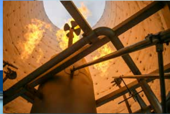
↓ Propane pilot burner in operation
