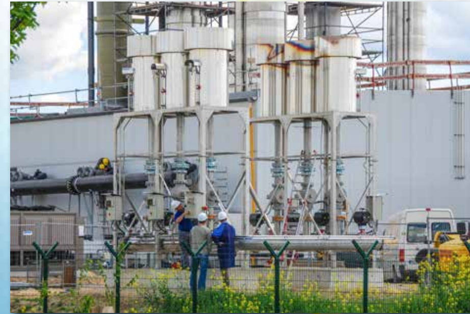
↑ Bivalent flare at Güstrow 12.000 m 3 /h biogas and 6.000 m 3 /h biomethane
