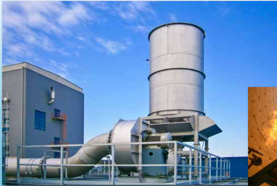
← Flare system for 30.000 m 3 /h styrol steam incl. 13.000 litre propane gas tank with control station and 80kW emergency generator
